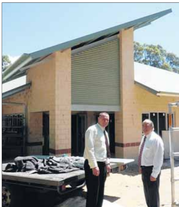
John views progress on the new administration building at Withers Primary School with principal Stuart Cumming.
