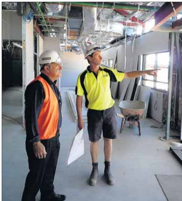
Bunbury MLA John Castrilli looks over progress on the new South West radiotherapy centre with Perkins site manager Ray Comley.
